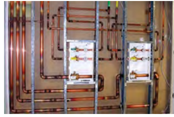
Medical Gas Pipeline
