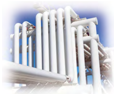
Industrial Gases Pipeline
